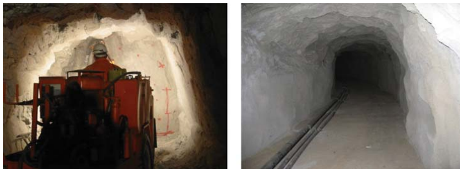
Figure 9. The dilution supply tunnel under construction (on the left) and completed (on the right).
